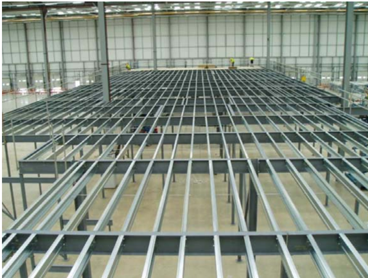
Phase I in progress: Davicon's floor for Knapp Logistik Automation at John Lewis' distribution centre
